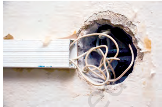
Fig. 1.28: Be careful of exposed cables
